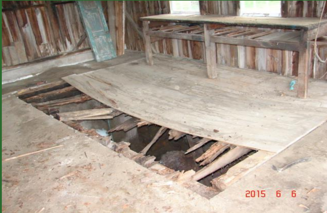
Dangerously collapsing wellhouse floor
