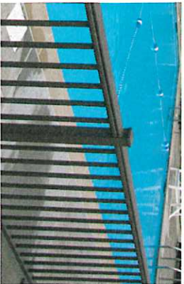
FENCE SURROUND AROUND WADING POOL IN COORDINATING COLOR
